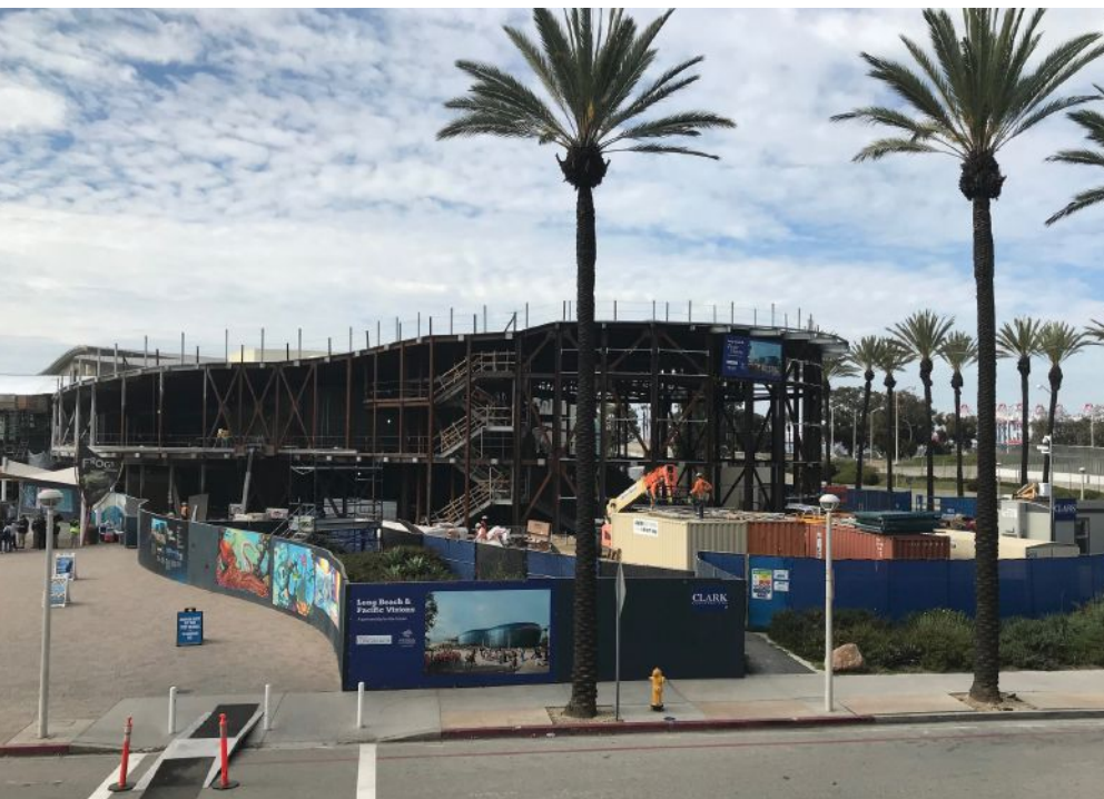
above and below: The framing for the addition used 350 tons of structural steel and 4,831 connection bolts to hold it all together—all delivered from North Dakota to Long Beach in 30 truckloads.
